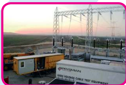
Prysmian HV Test Equipment
