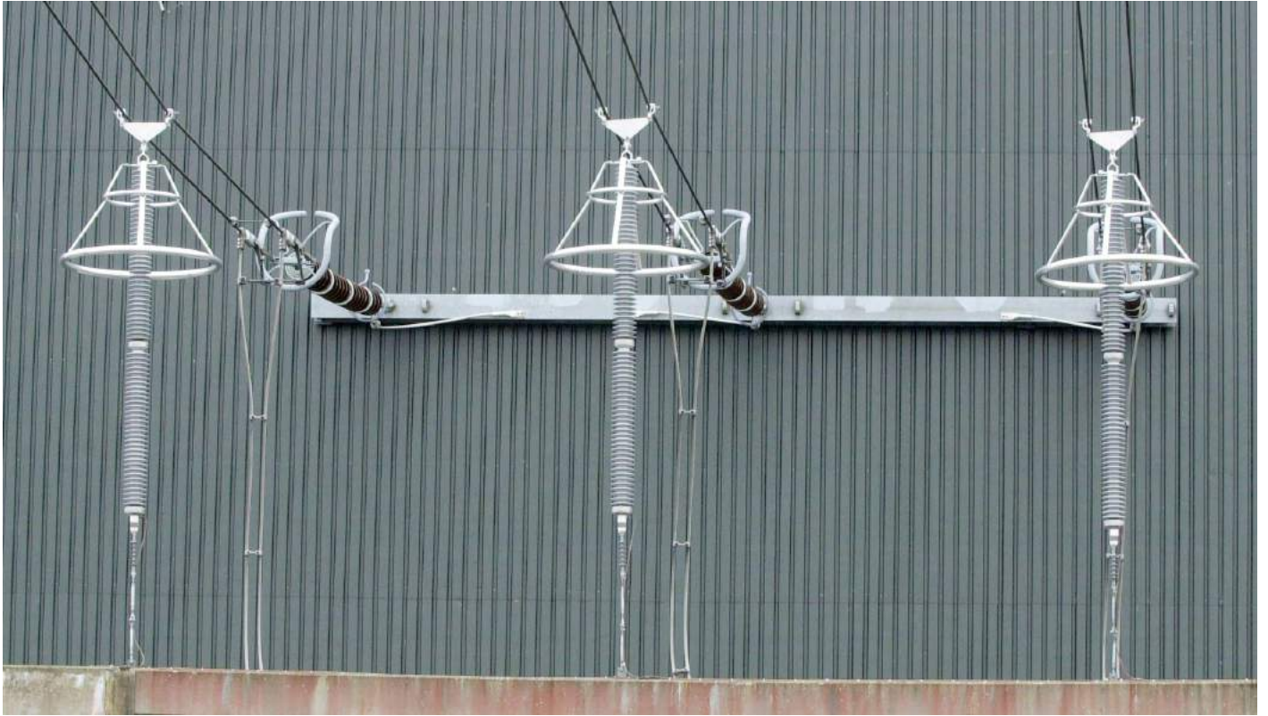
PEXLIM surge arresters connected to the 420 kV the secondary winding on a step-up transformer in a nuclear power plant
