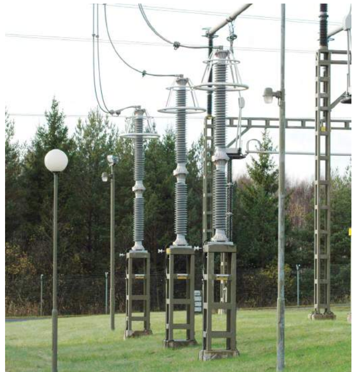
TEXTLIM surge arresters connected to the line entrance
