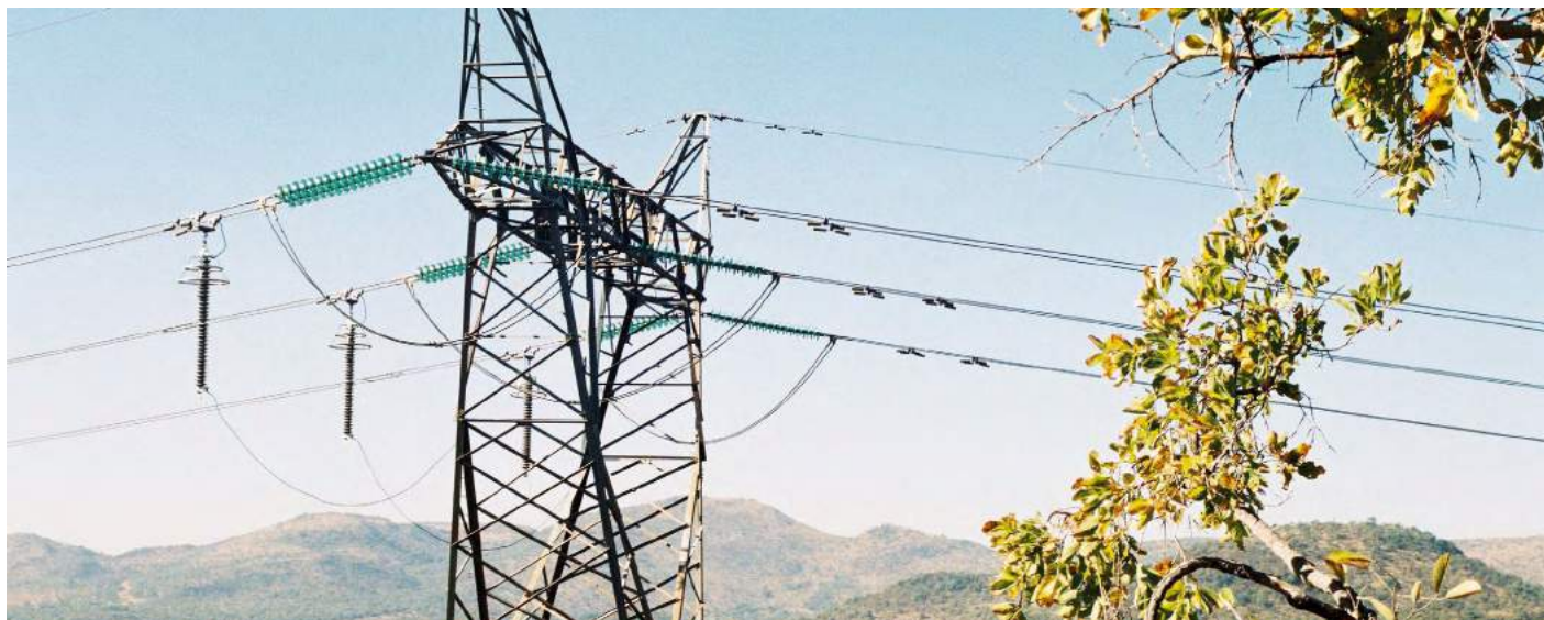
Line surge arresters, incorporating PEXLIM Q arresters and disconnecting devices on earth leads, erected on ESKOM 300 kV system in South Africa.
