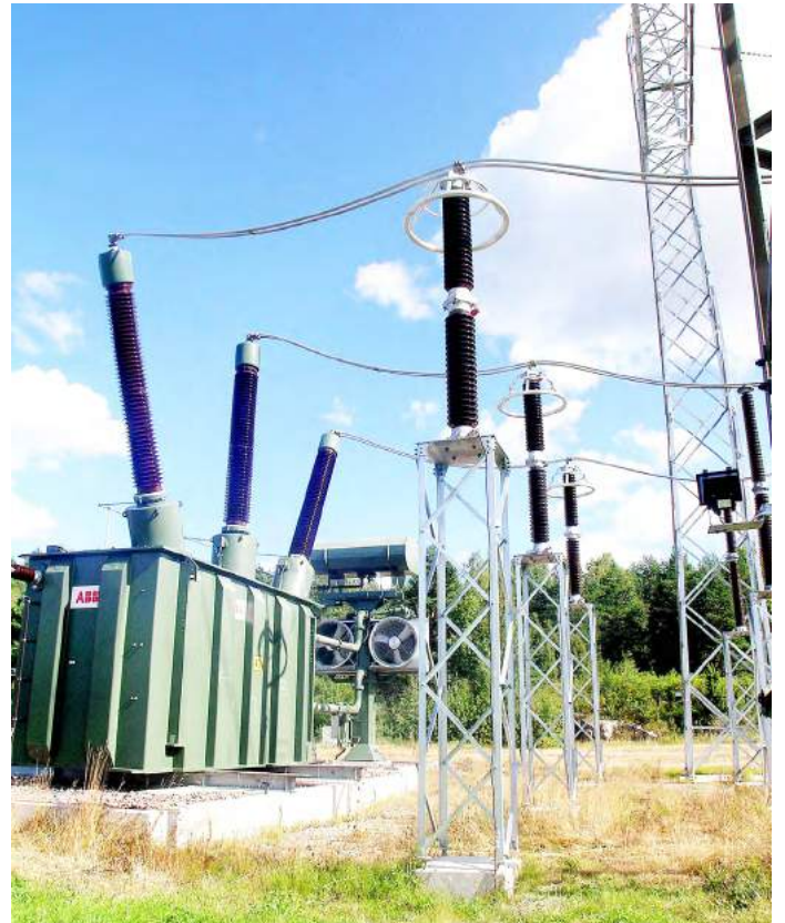
EXLIM surge arresters protecting a 420 kV power transformer
