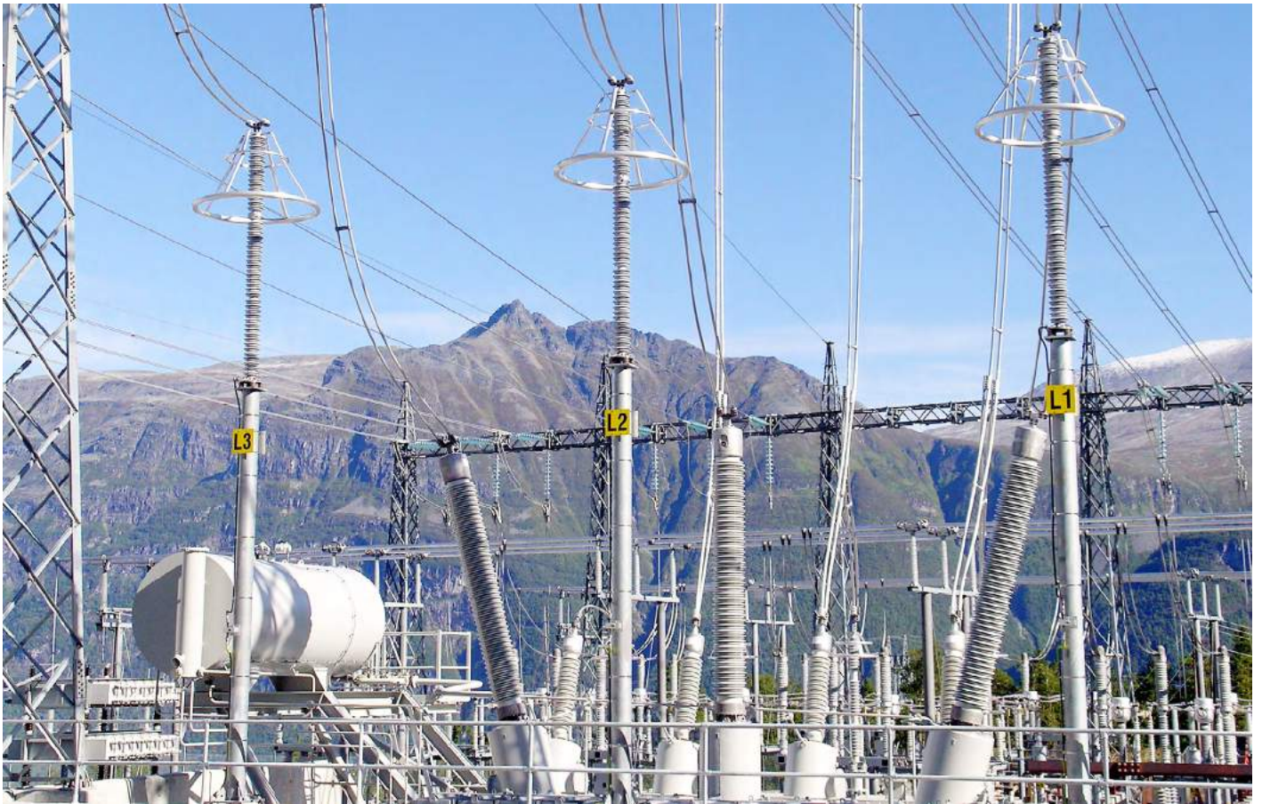
PEXLIM surge arresters protecting a 420 kV power transformer in Norway
