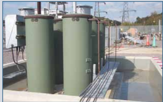
Outdoor Tank Farm
