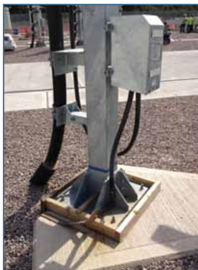
Gantry mounted link box
