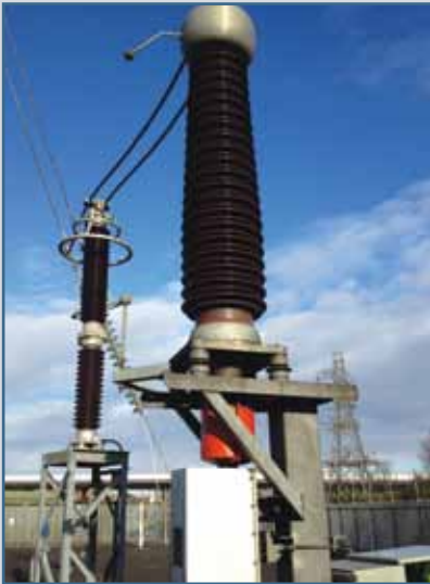
Outdoor Sealing Ends
