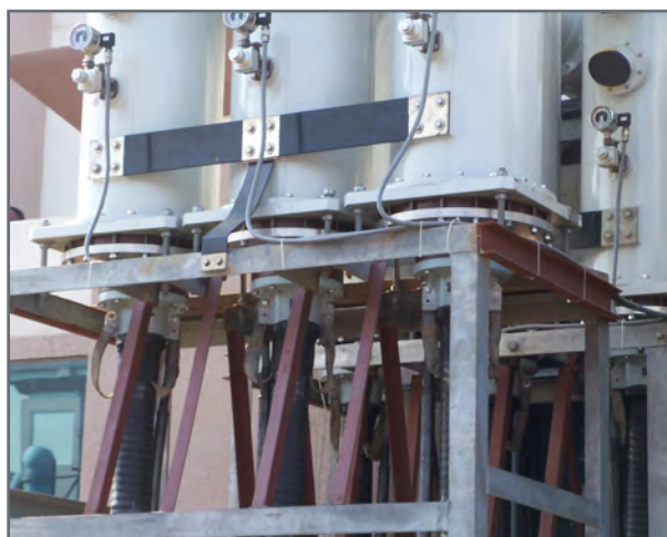
▲ PATR140-SF terminations installed in a GIS.
