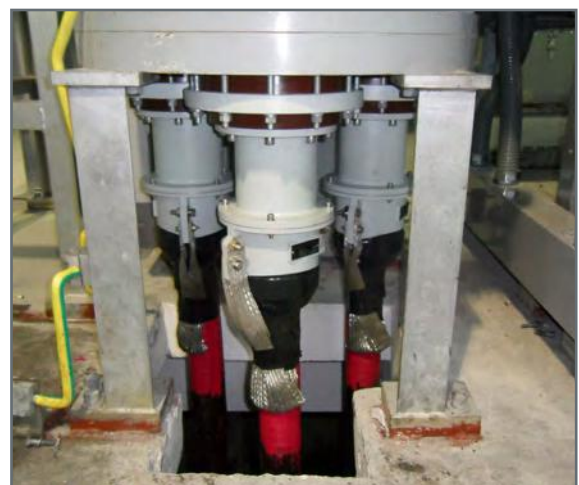
▲ SSC140-SF terminations installed in a GIS.
