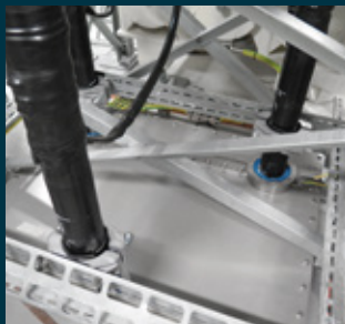
5. High voltage cables
