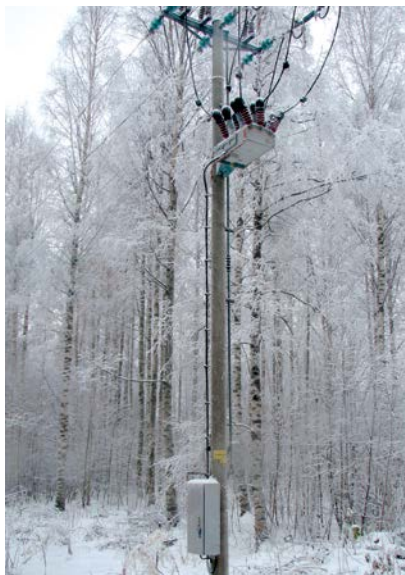
OSM RECLOSER AND CONTROL AND COMMUNICATIONS CUBICLE
