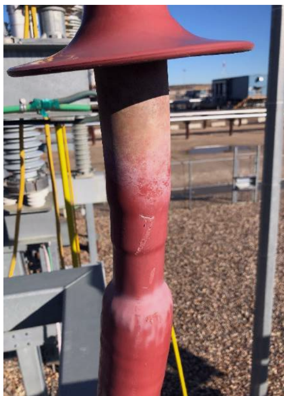
Cable termination H3 with uneven contamination
