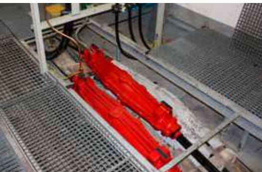
Oil refill joints in switch gear station
